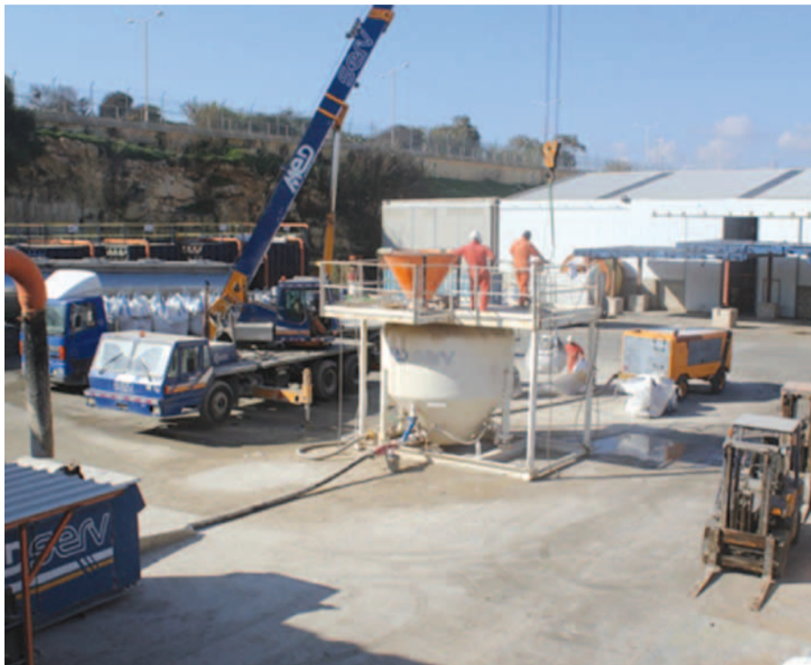
The mud mixing operation at the Malta base which was recently completed for a leading American company operating in Tanzania.
