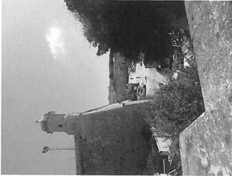
Fig: 26 Present condition of outerwork ditch to be upgraded#
