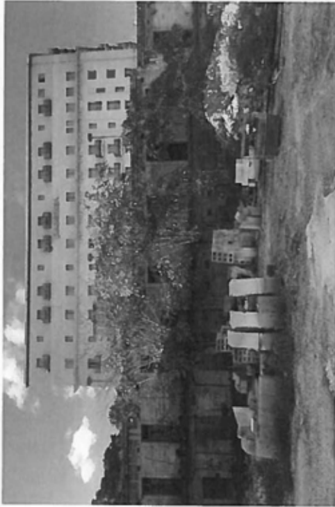
Fig: 27 Present condition of outerwork ditch to be upgraded
