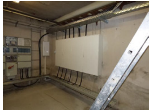
Current meter cabinet
