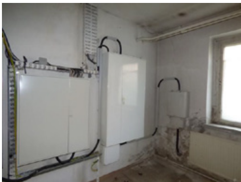
Current meter cabinet
