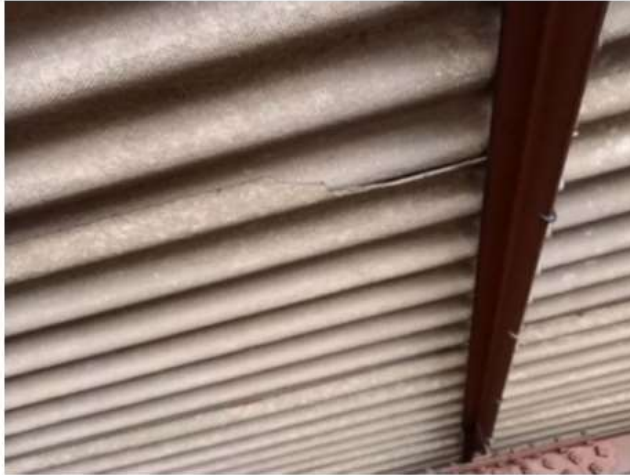
Pic 23 Internal view of roofing structure showing deterioration
